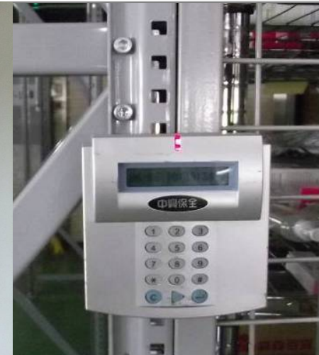
RFID Protected Doors
